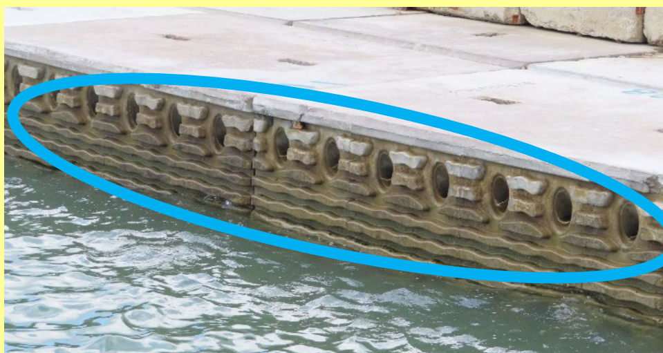
Example: Vertical Eco-shoreline at Tung Chung (eco-tiles)
